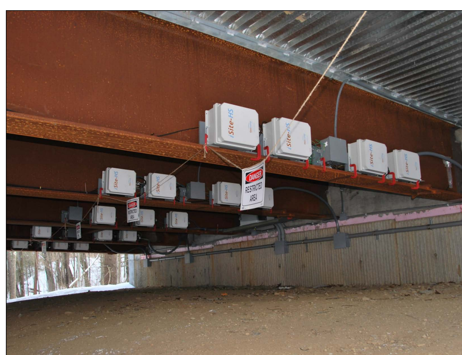
Fig. 3 Data acquisition units under Vernon Avenue Bridge
